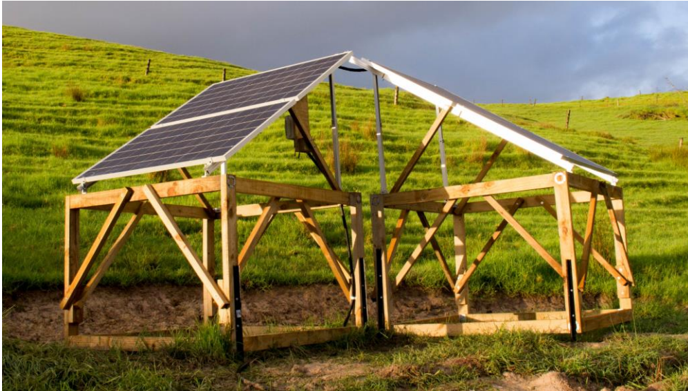
Typical installed PV array
